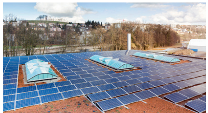
Figure 7: Photovoltaic facility (© Biogas Zürich)
