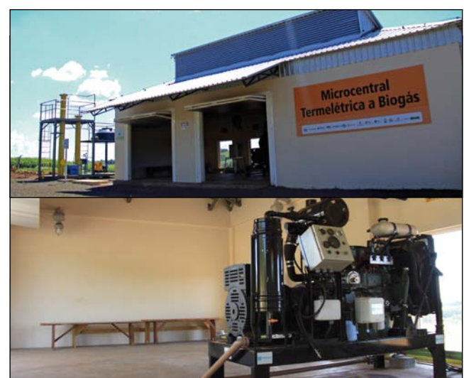
Figure 4: The centralised combined heat and power (CHP) plant supplied by biogas through the biogas pipeline
