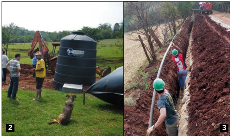
Figure 2: A anaerobic digesters for biogas production during installation on small farms included in the project
