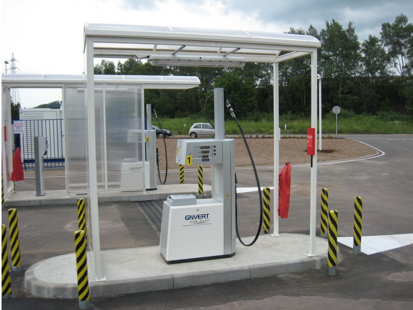
CNG filling station (Forbach)
