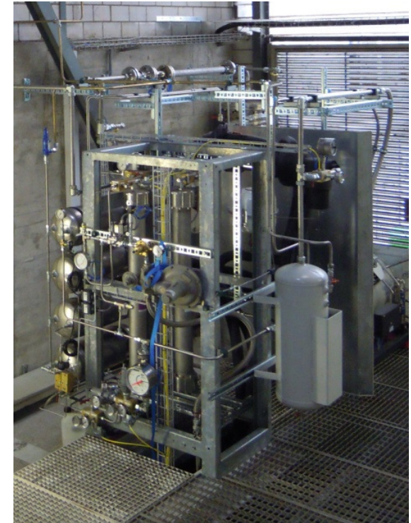
Blue BONSAI BB15, installed at an industrial biogas plant
