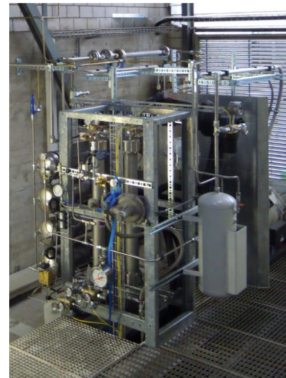
Blue BONSAI BB15, installed at an industrial biogas plant
