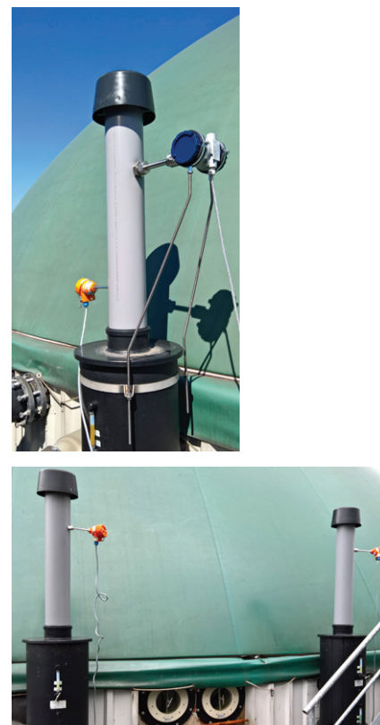
Figure 16: Measurement setup for PRV monitoring (DBFZ)
