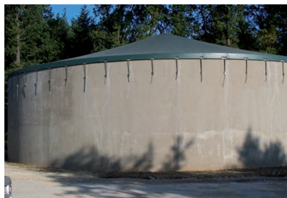
Photo 5: Covered digestate storage tank
