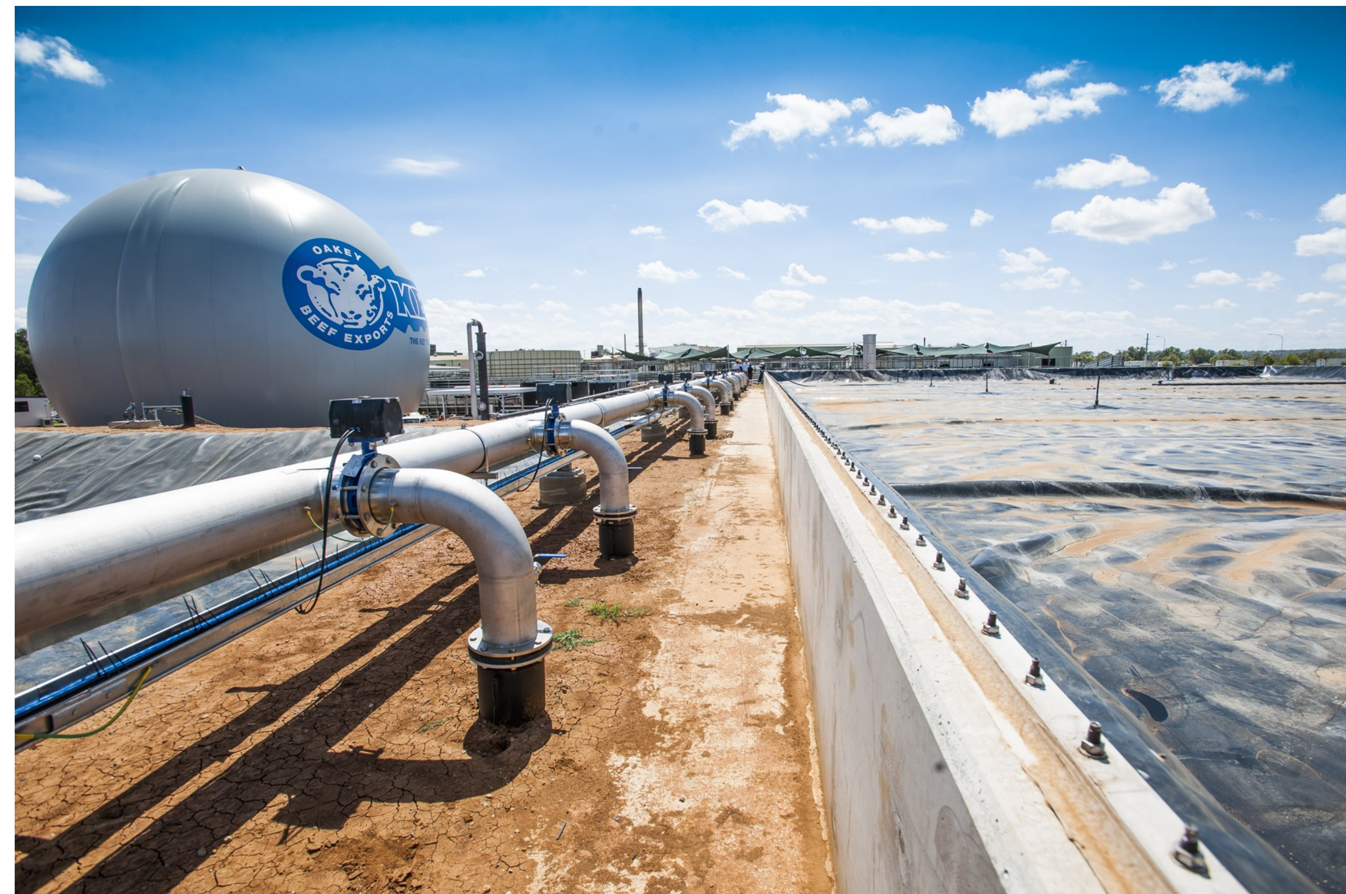
Figure 2: Example of a covered anaerobic lagoon treating abattoir wastewater
