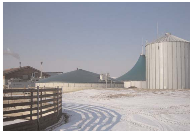
Figure 1: The "Rohkraft" Biogas plant in Reidling, Austria. From left to right the CHP unit, the covered digestate storage tank, the second digester step with gas cover and a gas storage tank can be seen.
