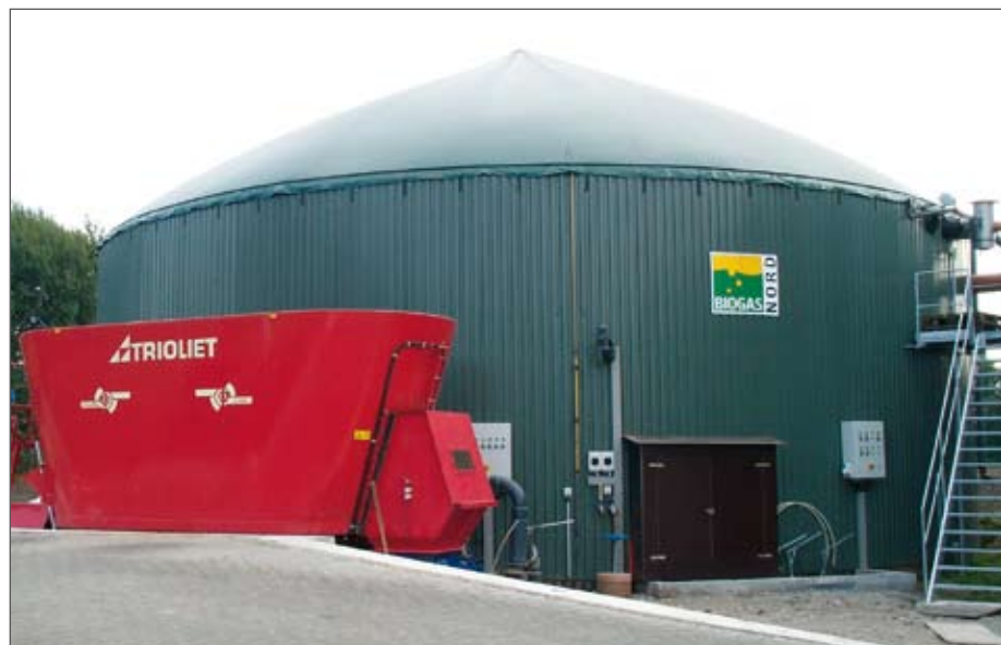
Photo 1: Anaerobic Digestion plant in Germany
