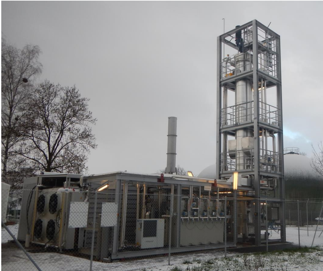
Figure 15.1. Aarmatt Biomethanation plant, Store&Go Project
