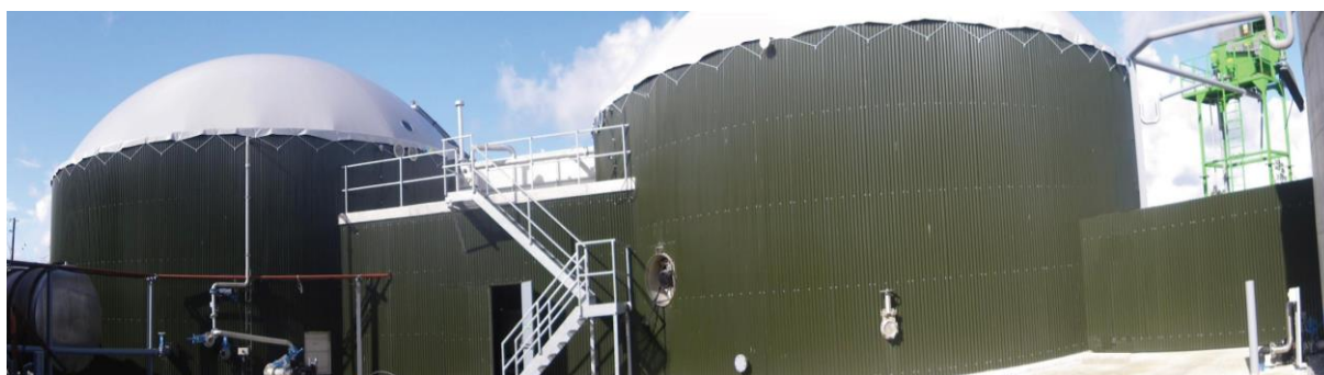
Figure 12.1. Biogas plant McDonnell Farms Limited. Primary Digester and first covered storage digester. David McDonnell milks 300 dairy cows in Limerick and also operates a free range poultry farm. In 2009/2010 he installed the most modern farm digester in Ireland which has a capacity of 250 kWe. (Source: SEAI (Sustainable Energy Authority of Ireland) Anaerobic Digestion: A case study – McDonnell Farms Biogas Limited, Shanagolden, Co. Limerick))
