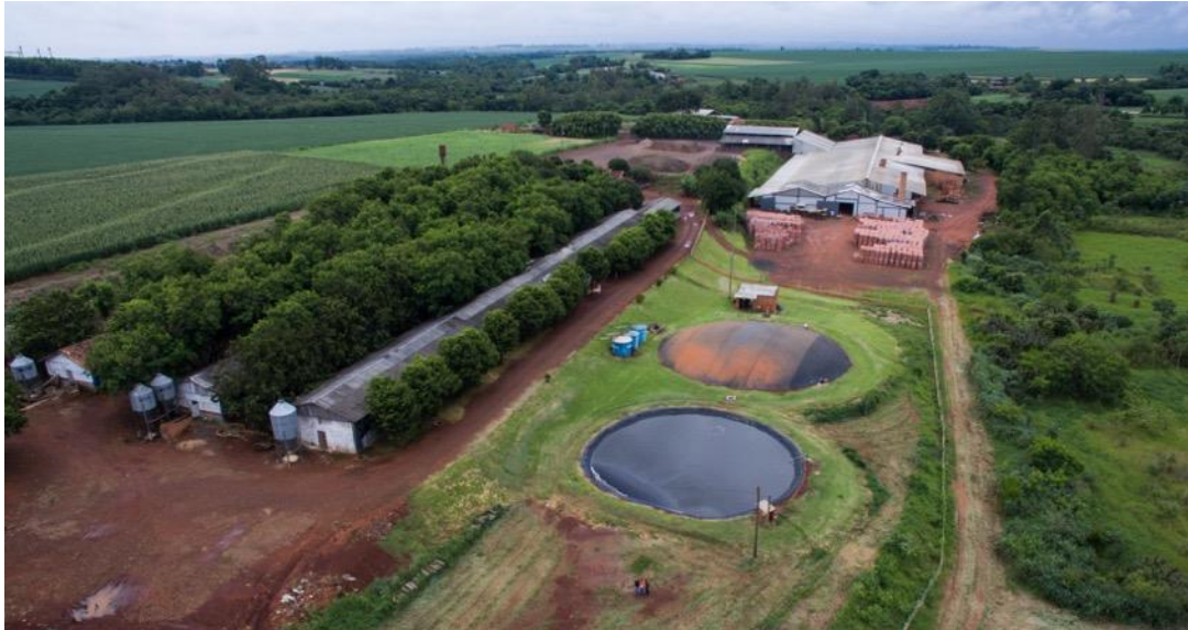
Figure 5.1. Stein Ceramics biogas plant
