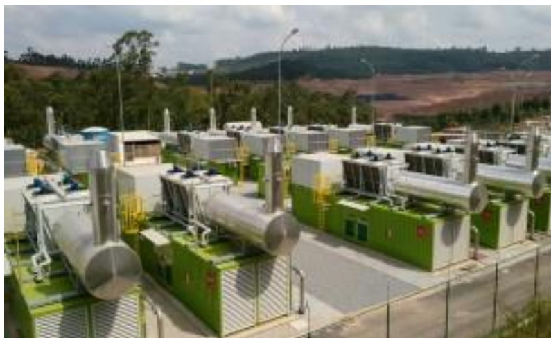
Figure 5.2. Termoverde Caieiras biogas power plant
