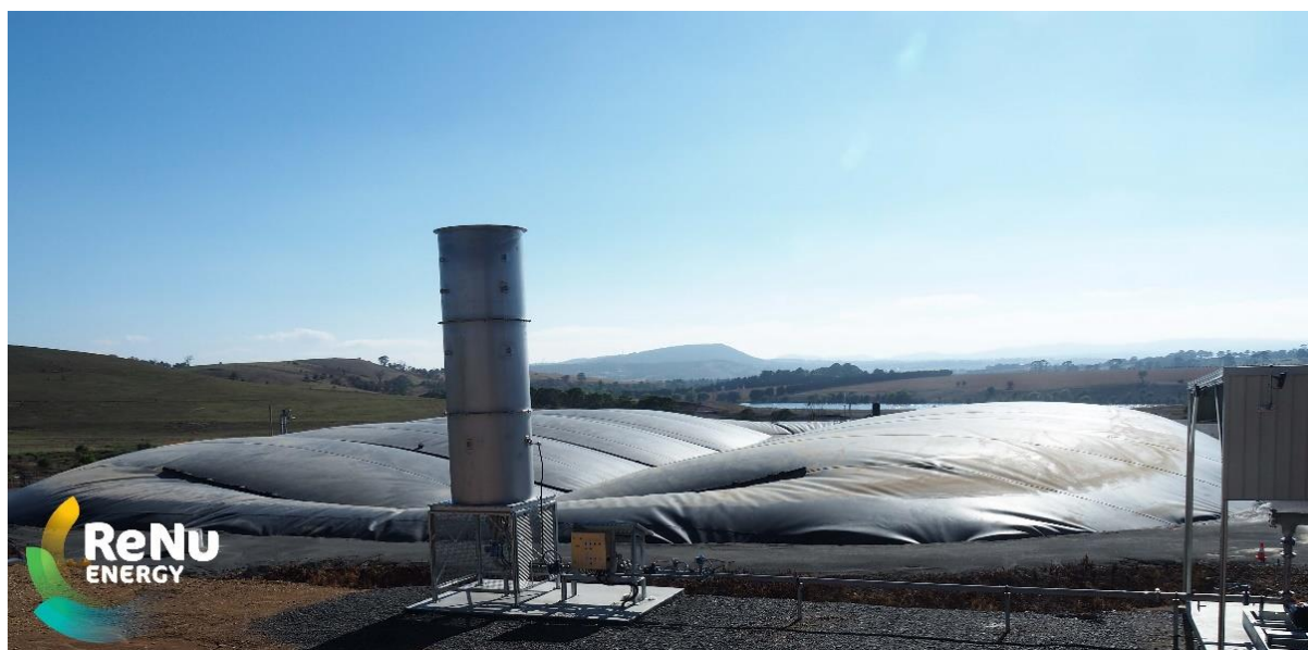
Figure 3.1. Anaerobic digester and flare of the Goulburn Bioenergy Project (photo: ReNu Energy) 7
