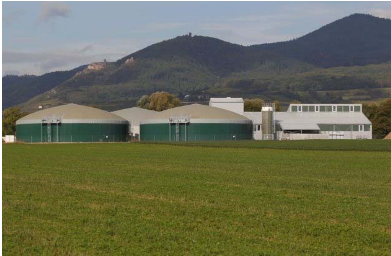
Centralised plant AGRIVALOR (Ribeaupillé, Lorraine) 26 000 tons capacity 1400 kWe and district heating system for a casino's swimming-pool
