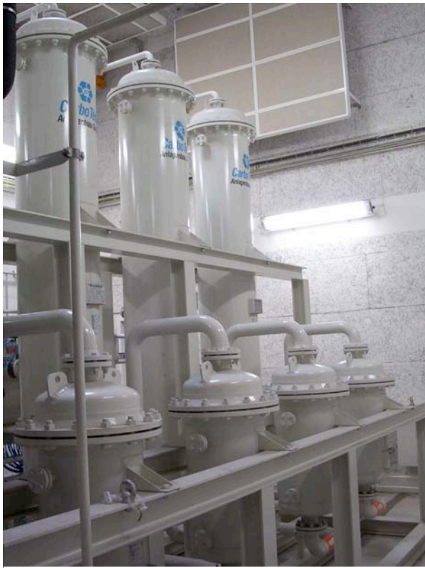
350 m 3 /h upgrading plant with PSA-technology Helsingborg, Sweden
