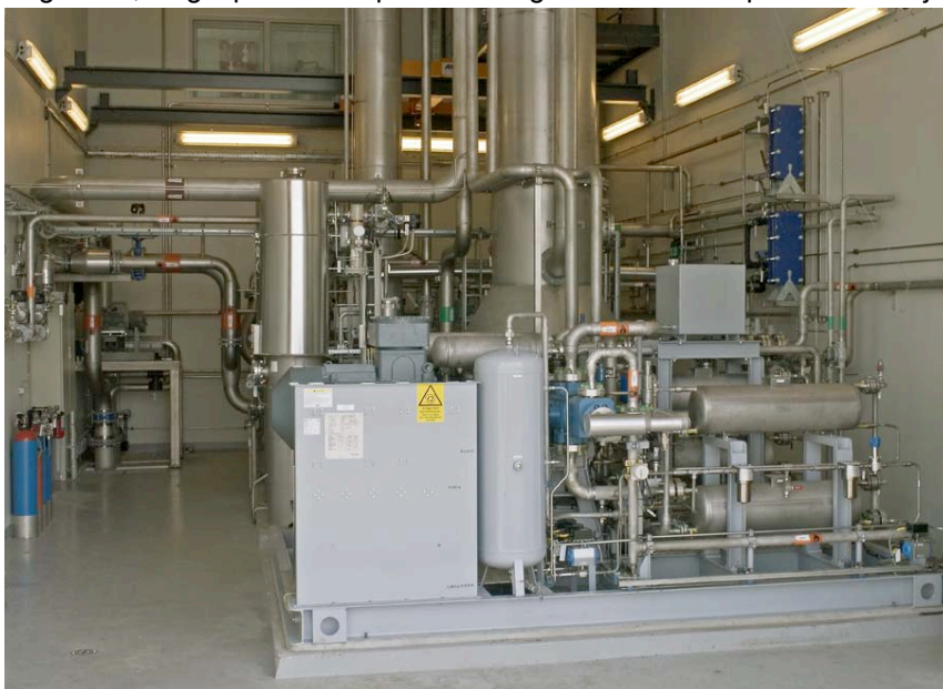
600 m 3 /h upgrading plant with water scrubber technology Henriksdal sewage water plant, Stockholm
