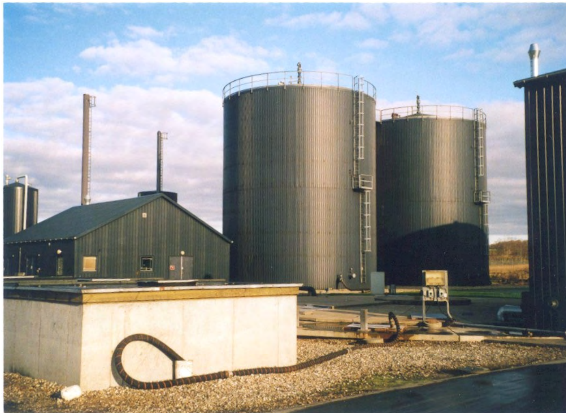
Central digester in Studsgard
