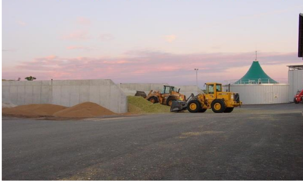
Maize silos, digester and gas storage of the Energy Crop Digestion Plant Reidling
