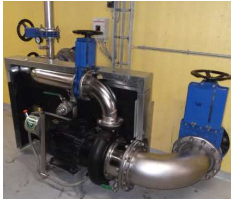
Sludge Mixing- and Treatment
