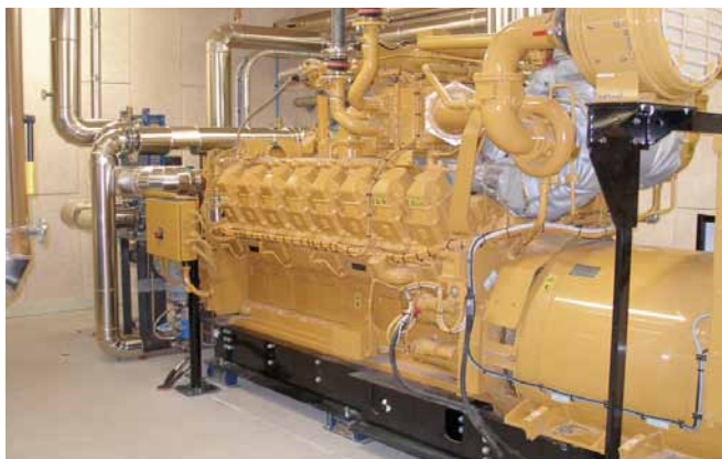
Figure 5: Caterpillar 3516, 1121 kW, at the biogas plant in 2010 (Photo: Linko Gas)
