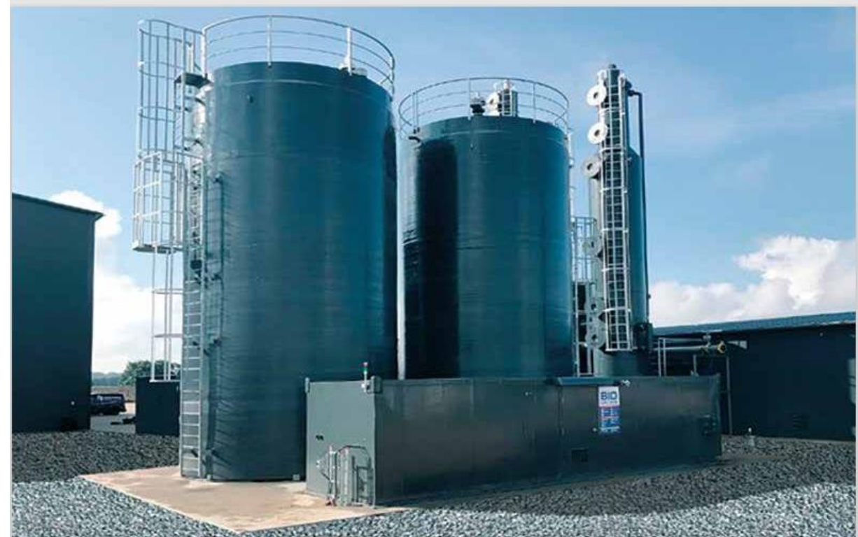
FIGURE 5.4 Biogascleaner QSR desulphurization plant at Nature Energy Maansson in Brande, Denmark. PHOTO Biogasclean.
