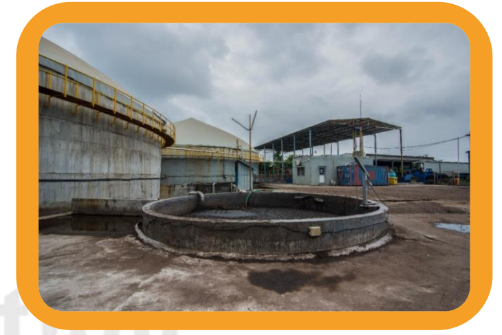
Large Scale Biogas Plant (>2500m 3 )
