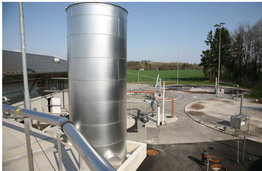
Figure 7 Biogas plant at the slaughterhouse in St. Martin, Upper Austria
