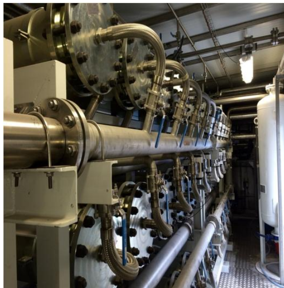
Figure 14 Membrane technology (reproduced with the kind permission of AGRANA)
